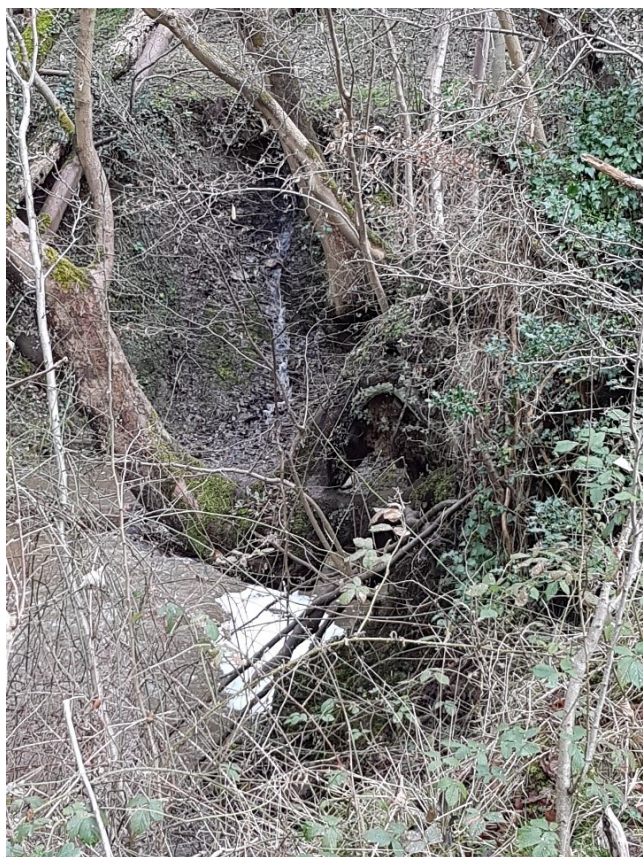
Seepage through made ground creating small waterfall
